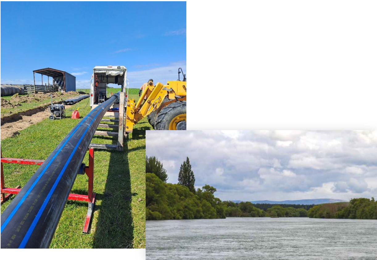
Figure 2-6 Pipe welding and installation (left) as part of the Greenfield Water Scheme Project which will link from the lower Clutha River (right) to Lawrence
