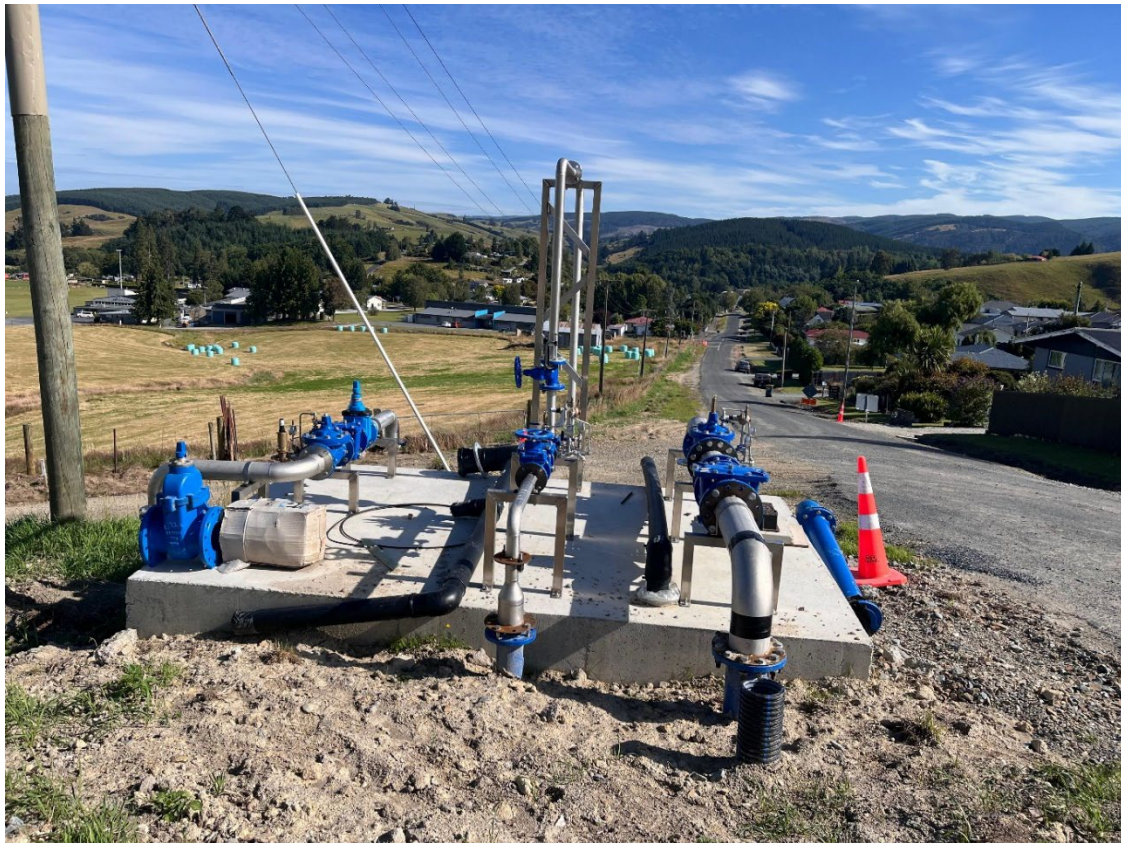
Lawrence pressure reduction valve (PRV)
