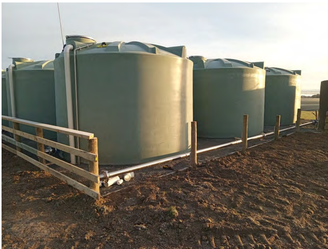
30m 3 Plastic Tank Farm Reservoir in Moffat reservoir, for reference only
