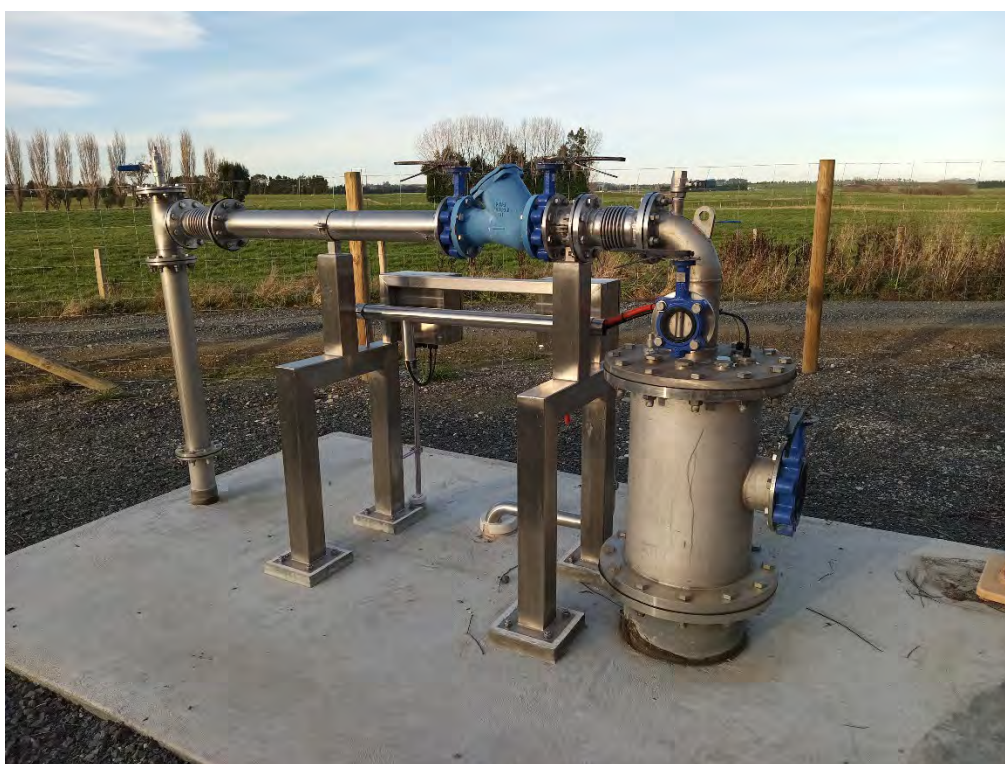
Installed Clydevale WTP Bore No.4, for reference
