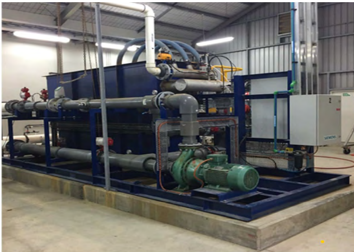
Milton WTP Membrane Unit No.1
