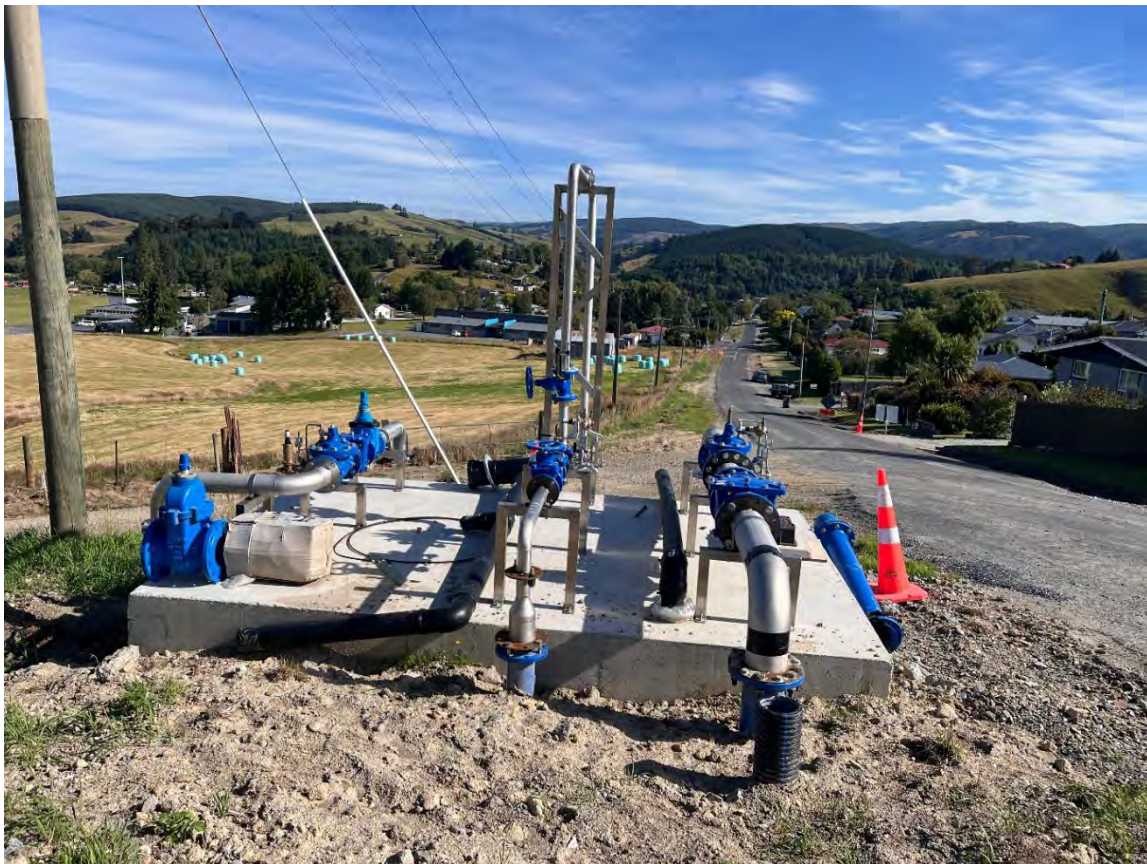
Lawrence pressure relief valve (PRV)
