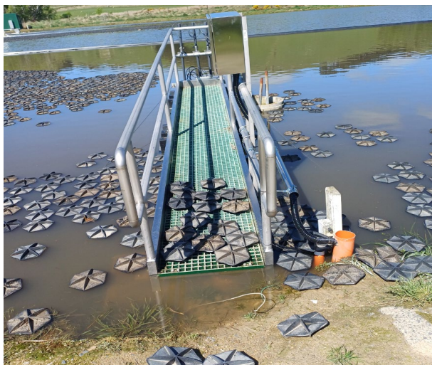
Hexcover on the gantry at Waihola WWTP
