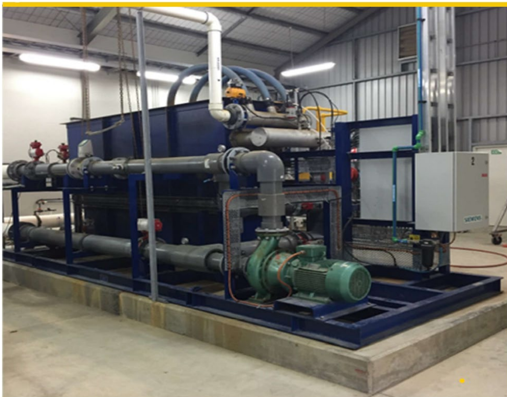
Milton WTP Membrane Unit No.1
