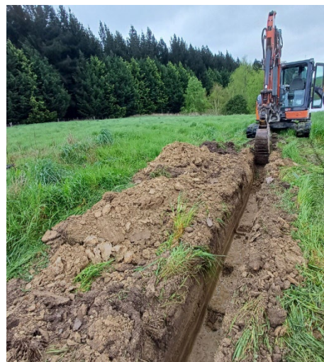
Screen waterline to setting Balclutha WWTP inlet
