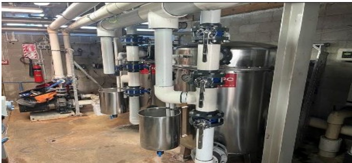
Balclutha Centennial Swimming Pool Perlite Filters
