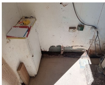
Mt Mistake Pump Station Interior
