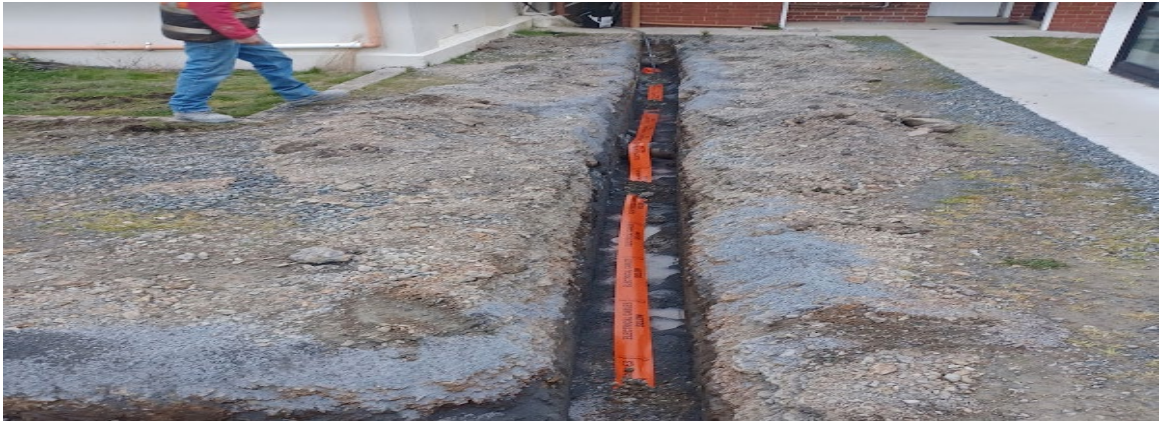
Inside property connection with power cable installed under crusher dust and warning tape on Union Street.
