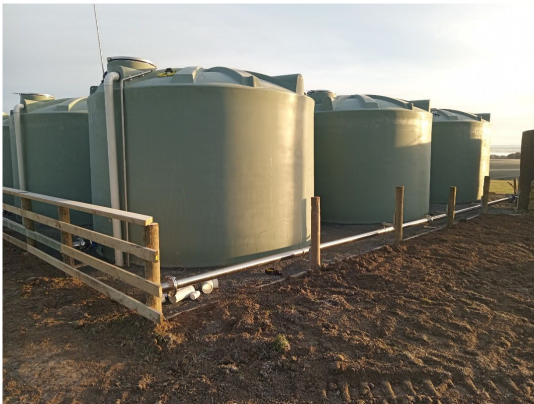
30m3 New Plastic Tank Farm Reservoir
