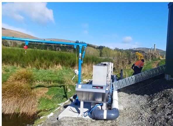
UV at Clinton Waste Water Treatment Plant.
