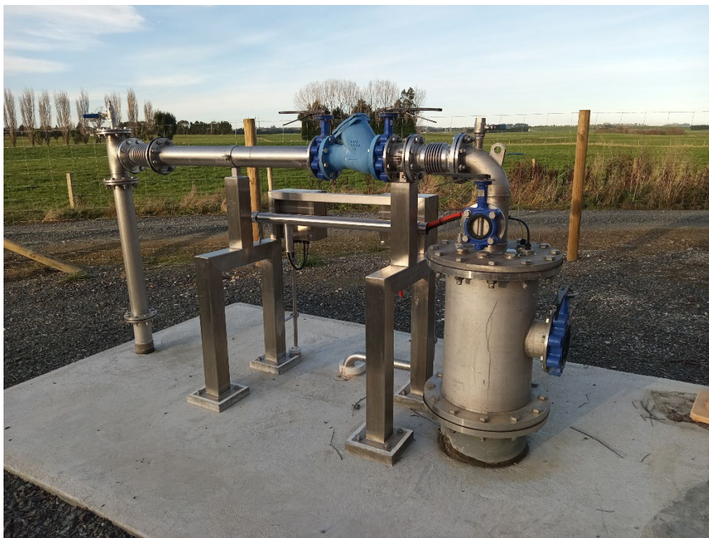
Clydevale WTP Bore No.4
