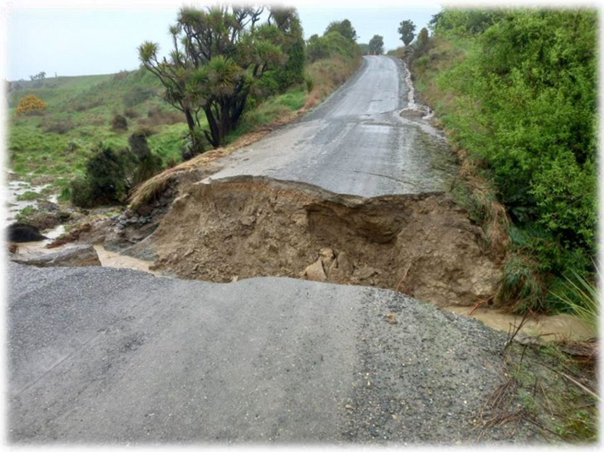
Summer Hill Road Washout
