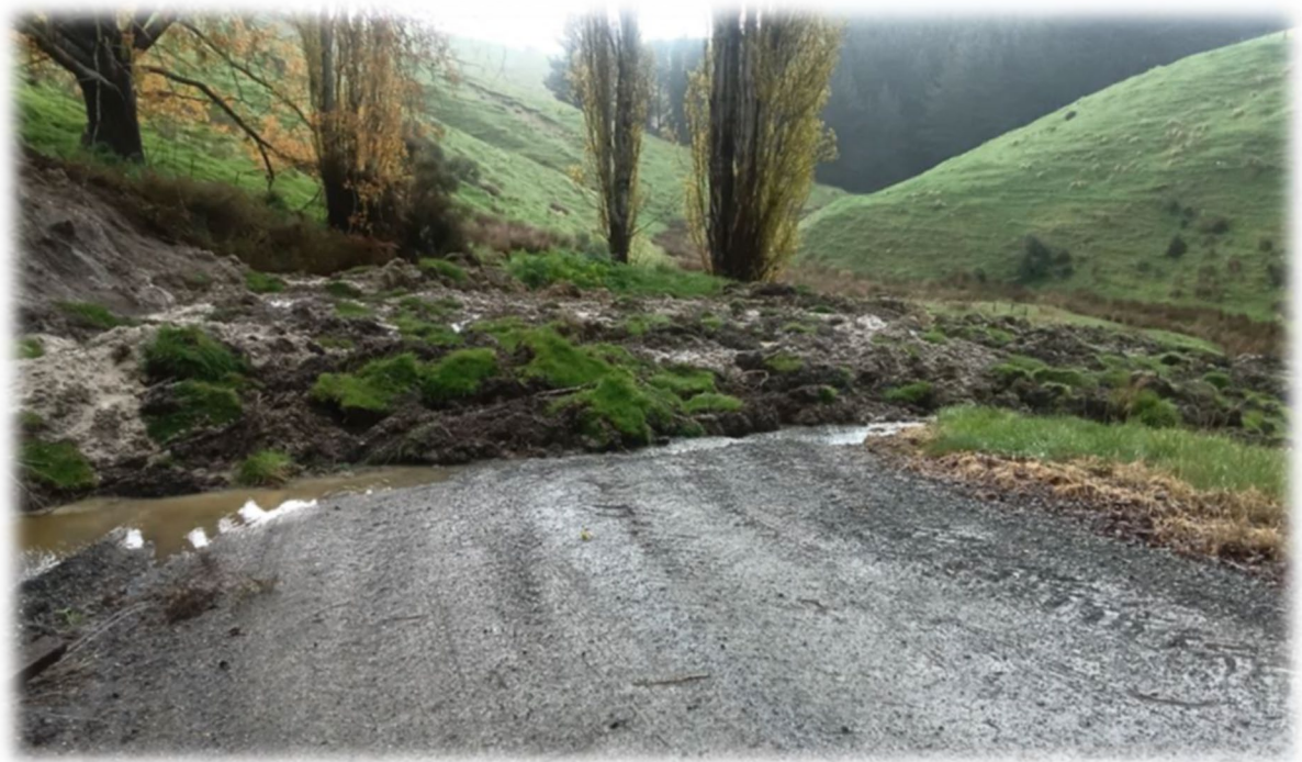
Wingfield Road Slip
