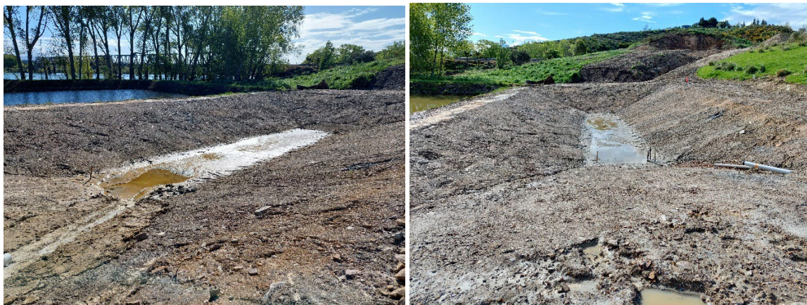
New leachate Pond Levels
