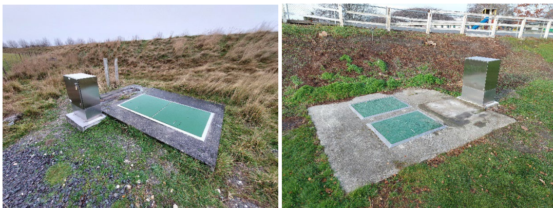
Stormwater Small Switchboard
