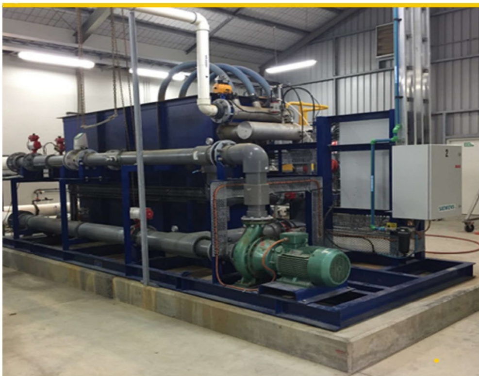
Milton WTP Membrane Unit No.1
