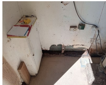
Mt Mistake Pump Station Interior
