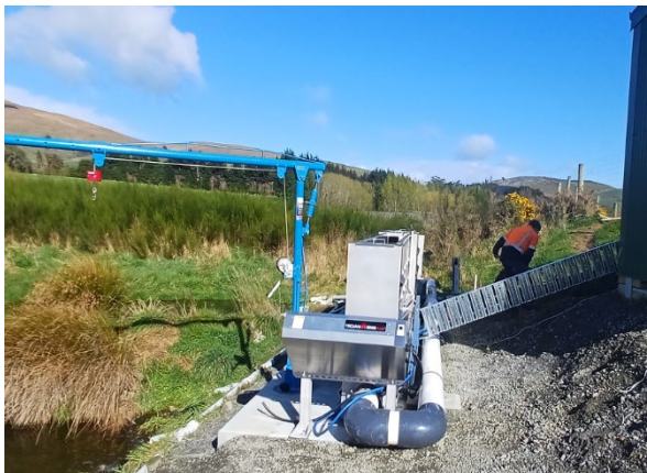
UV at Clinton Waste Water Treatment Plant.
