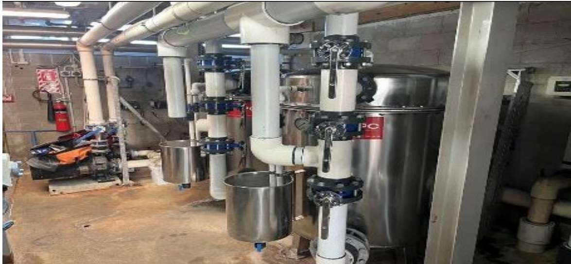
Balclutha Centennial Swimming Pool Perlite Filters
