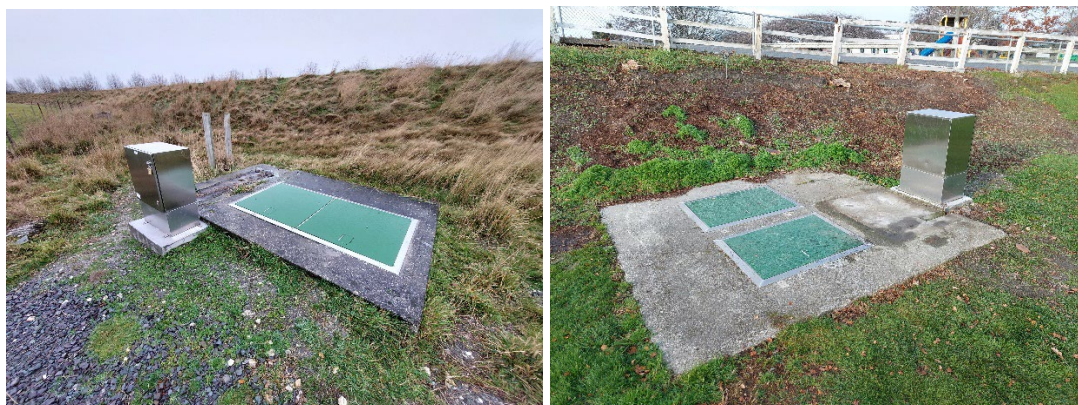
Stormwater Small Switchboard
