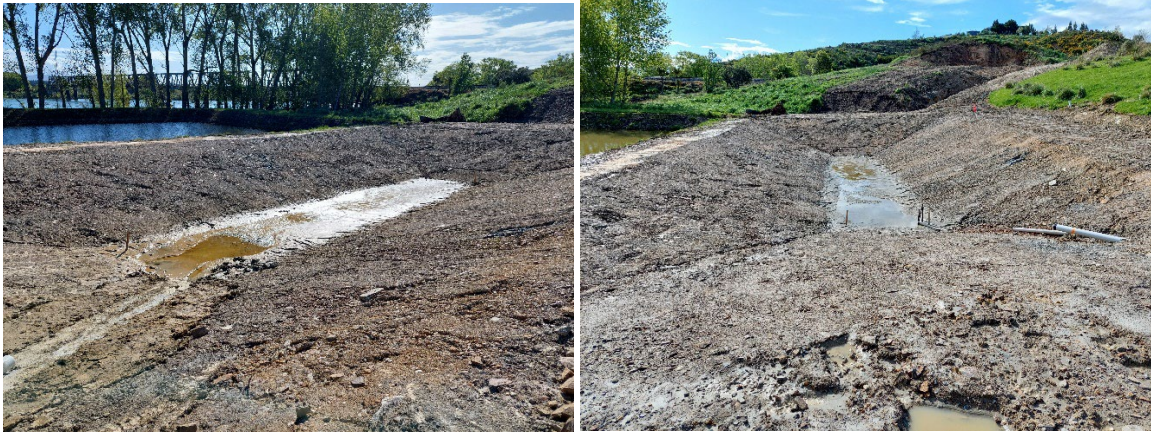
New leachate Pond Levels
