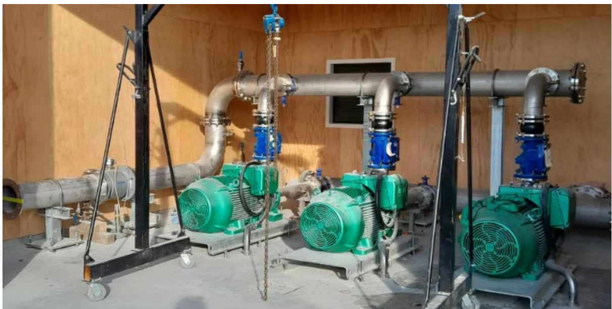
Photo 3 – Lower Greenfield Pump Station – pumps and pipework installed.
