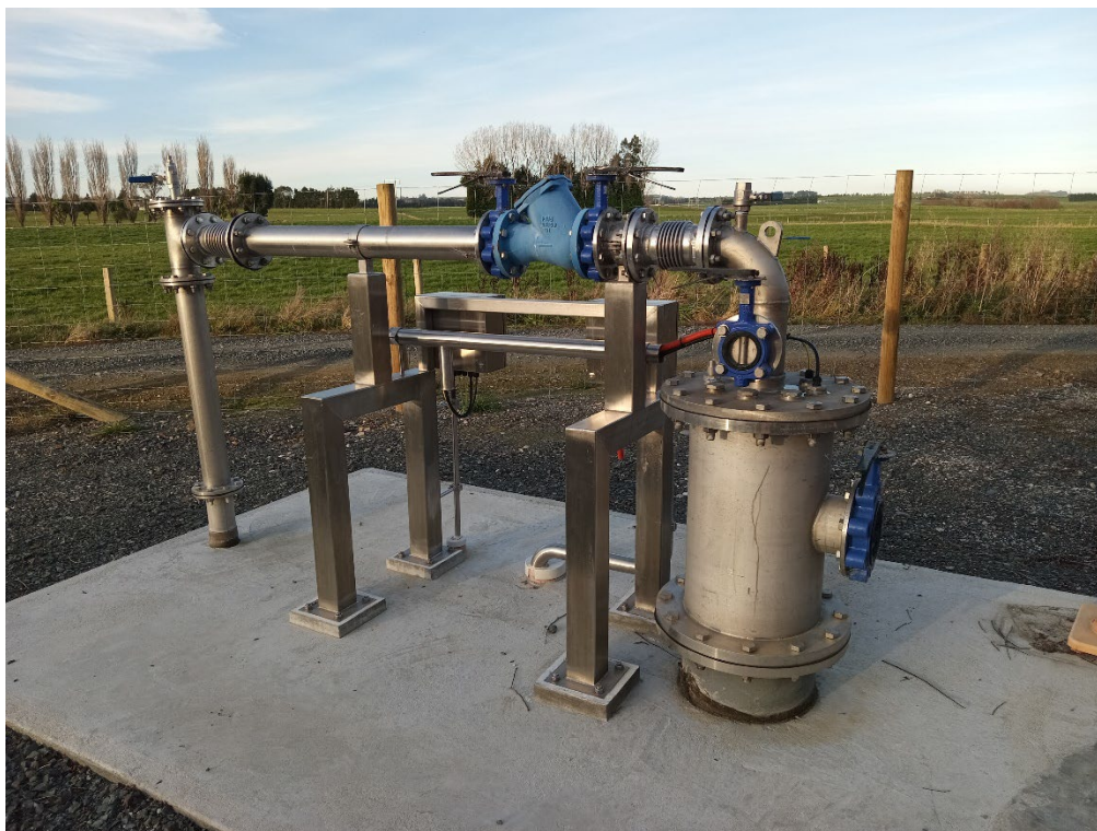
Clydevale WTP Bore No.4
