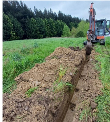
Screen waterline to setting Balclutha WWTP inlet
