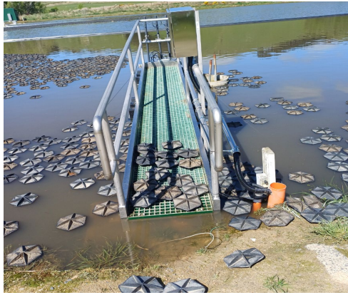
Hexcover on the gantry at Waihola WWTP
