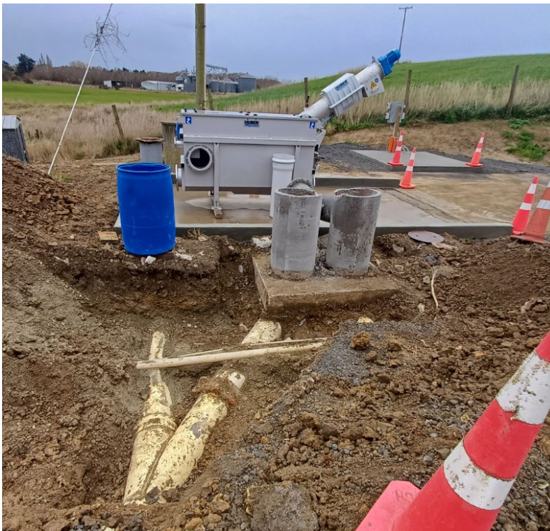
Inlet Screen at Balclutha Waste Water Treatment Plant
