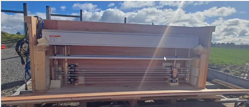
UV lights (already installed within the UV unit)
