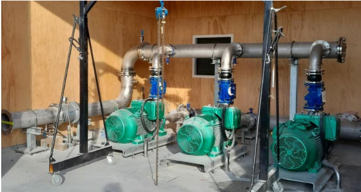
Photo 3 – Lower Greenfield Pump Station – Pumps and pipework installed.
