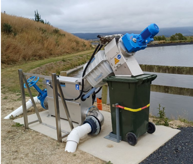
Inlet Screen at Waihola Waste Water Treatment Plant
