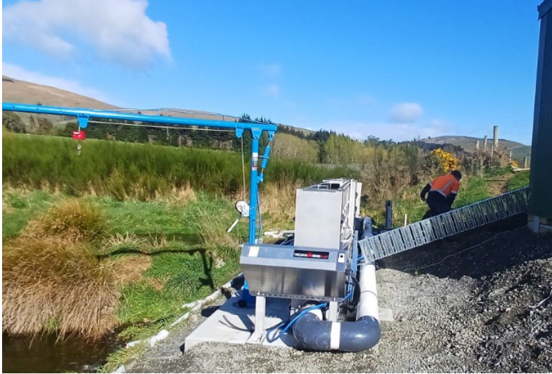
UV at Clinton Waste Water Treatment Plant.
